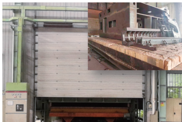
回火炉 / Tempering Furnace
